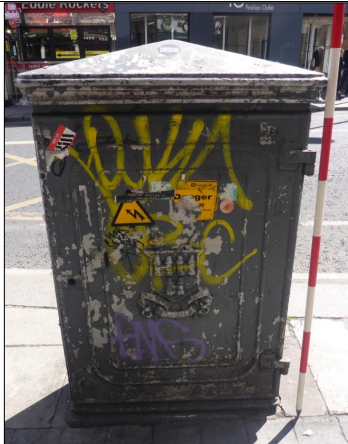
Electrical Cabinet on Wexford Street
