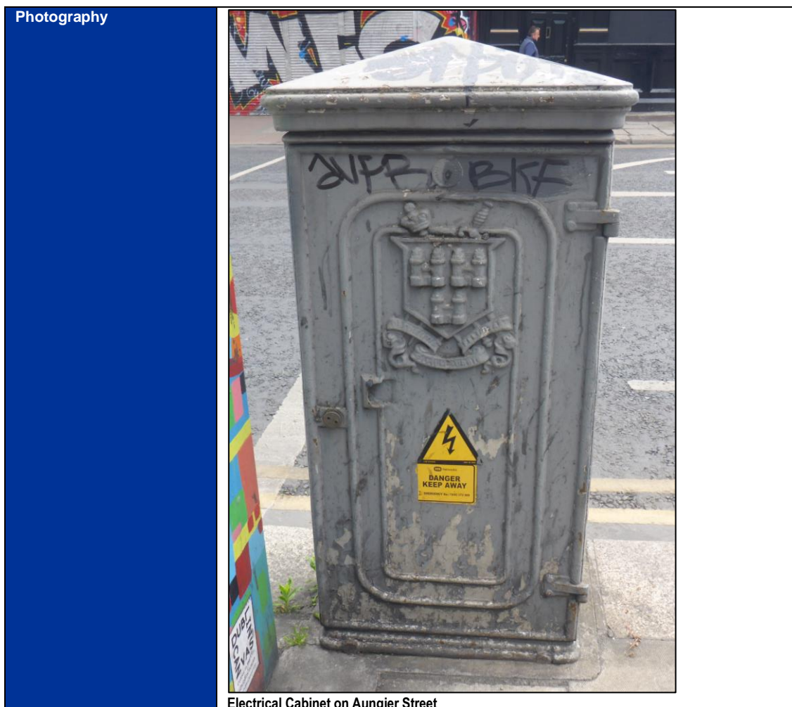
Electrical Cabinet on Aungier Street
